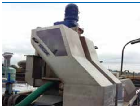
Waste water treatment plant (SEPCOM Industrial Vertical)
